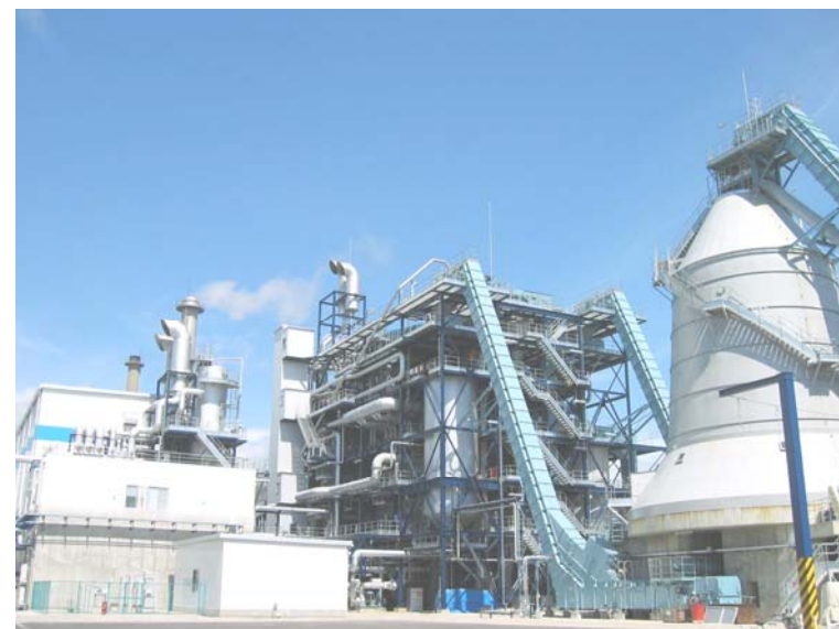
Thermal Recycle Power Generator (scrap wood fuel) at Nakoso mill
