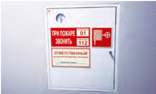
Fire extinguishing system installed inside an office
