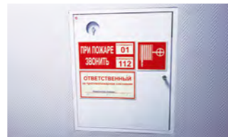
Fire extinguishing system installed inside an office
